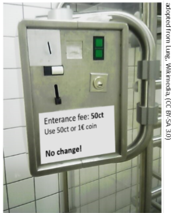
Fig. 11: Entrance Control for Toilets
